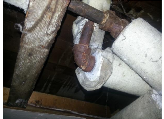
Random photo of some of the most dangerous kind of Asbestos
