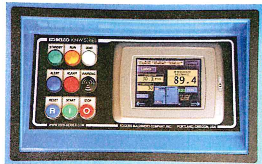
Figure 1-26 PLC operator interface and monitor. Source: Courtesy Rogers Machinery Company, Inc.
